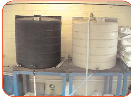
The pre-existing wastewater treatment plant at Beretta's Metal Finishing.
