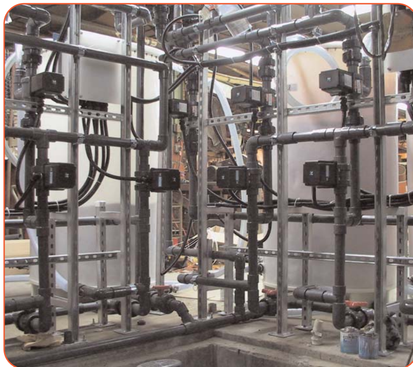
View of pipe manifold and tanks behind
