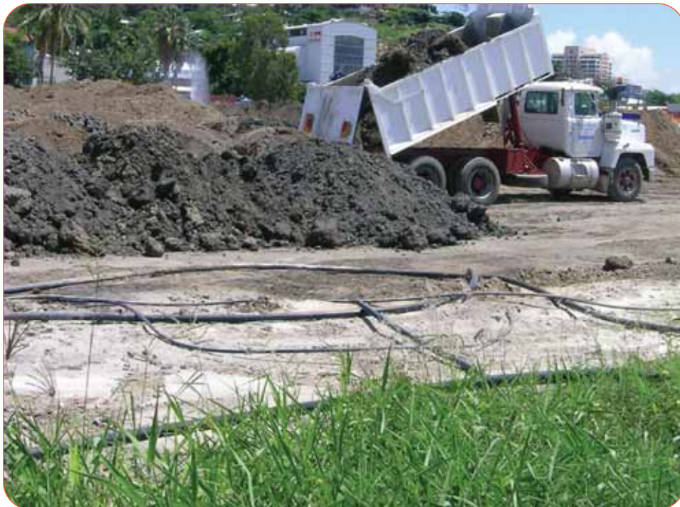
Figure 3 - Pouring contaminated soil into piles ready for the application of ViroSoil™ Technology with watering and aeration
