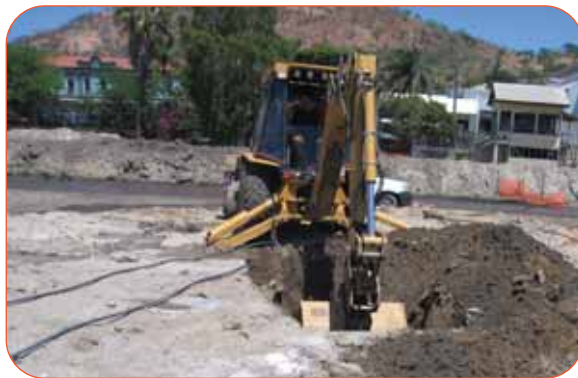
Figure 1 - Excavating the contaminated soil to be piled ready for treatment using ViroSoil™ Technology
