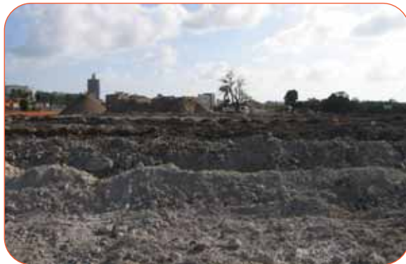
Figure 2 - Contaminated construction site before ViroSoil™ Technology application
